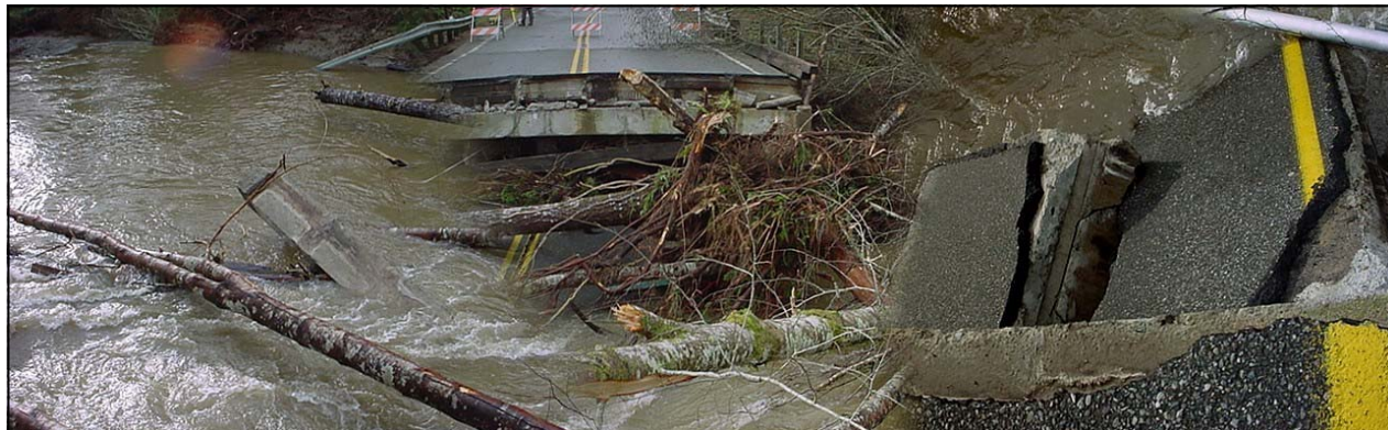
Photo courtesy of Hans Cregg, Mason County Public Works Dept. A Mason County road is literally swept away by water.
