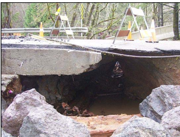
Mission Bridge in Mason County after the early December storm.
